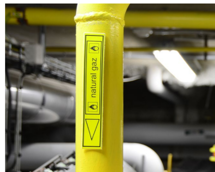
identification plates for piping or electrical circuits
