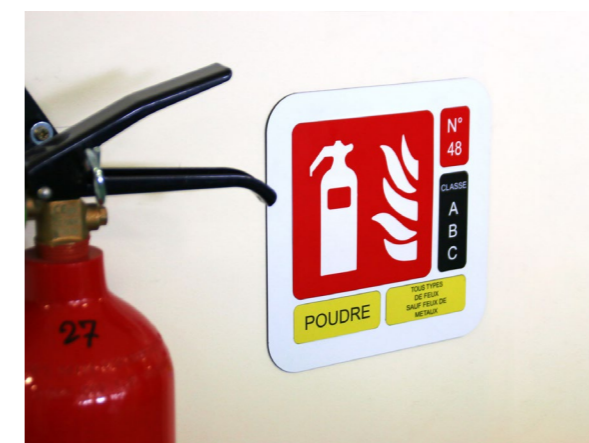
Pointing out safety features
